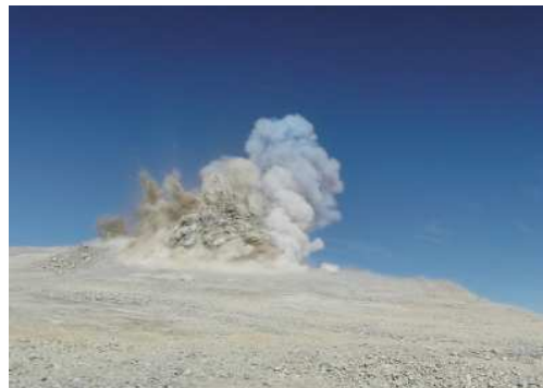
Fig. 2. The first blast on top of Armazones during the Ground Breaking Ceremony on June 19, 2014 marked the start of the site preparation activities that include the construction of a 25-km access road and the flattening of the top of the mountain.
